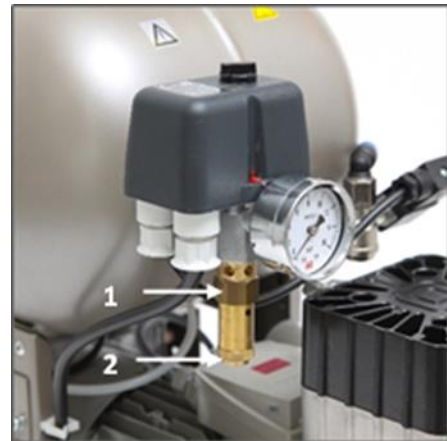
Fig. 7: Check of safety valve
