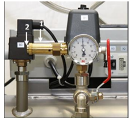
Fig. 17: Check of safety valve
