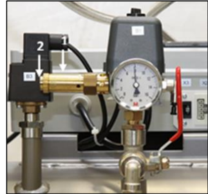
Fig. 25: Check of safety valve
