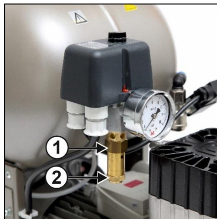
Fig. 13: Check of safety valve
