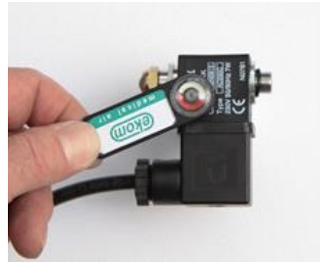
Fig. 28: Check of solenoid valve operation
